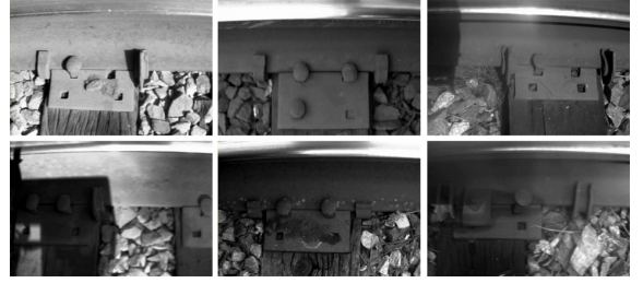
Fig. 7. Anchor appearance has a high variability due to the diversities in anchor type, size, shape, camera view, occlusion and lighting condition.
