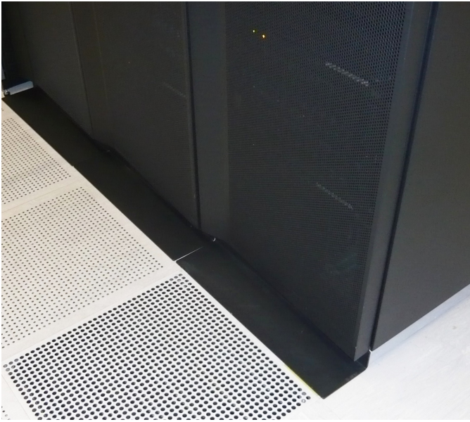
Fig. 8. Perforated floor tile was exchanged by one with bigger open area to provide more cold air to the rack at the location of node 40.
